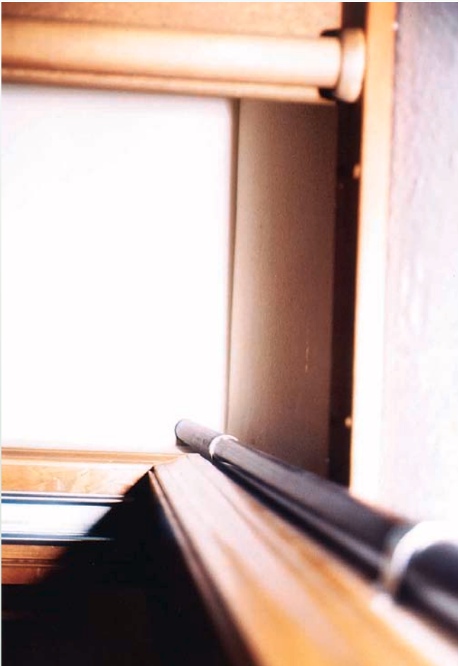
This hole we made in the ceiling for the conduit was the only interior impact our PV system had on the house.
