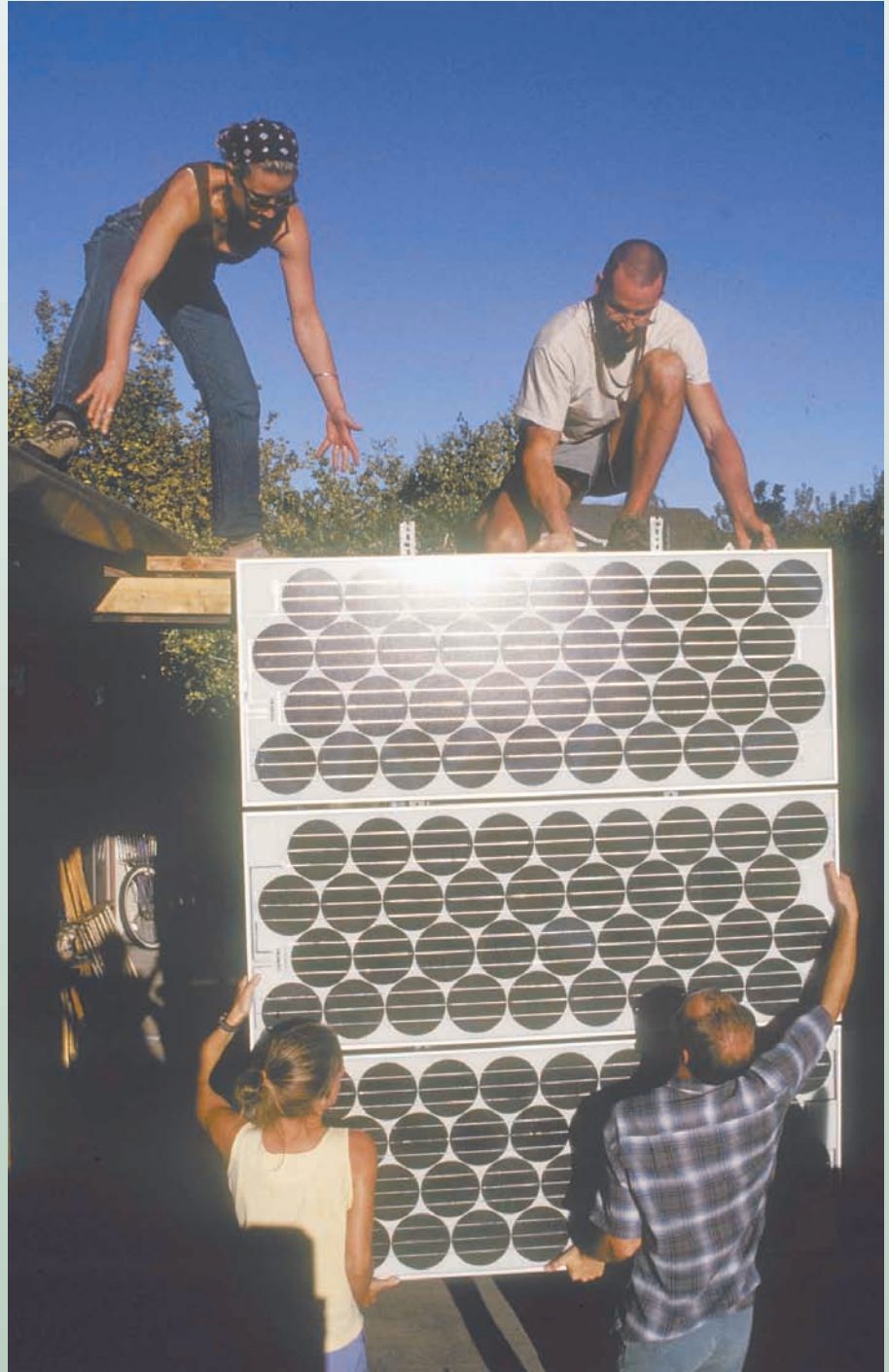
The de-installation crew lowers the rack and PVs—Tiffany, Scott, Nicole, and Scott. We designed the system to be easily movable because when you move a lot, what goes up, must come down.
