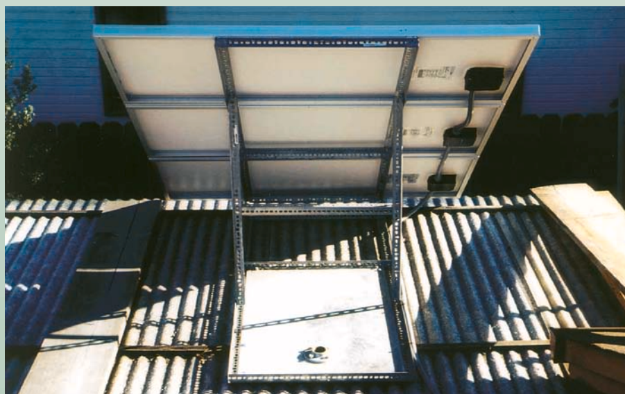
Six lag screws attached the PVs and homemade rack to the patio roof. After we de-installed the system (to move), we filled the holes with sealant and then put the screws back in.
